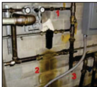
Leaks due to rust
