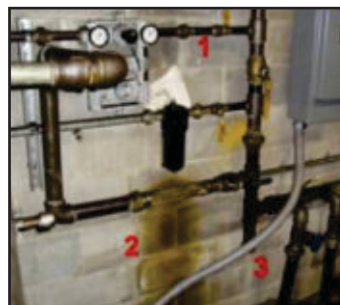
Leaks due to rust
